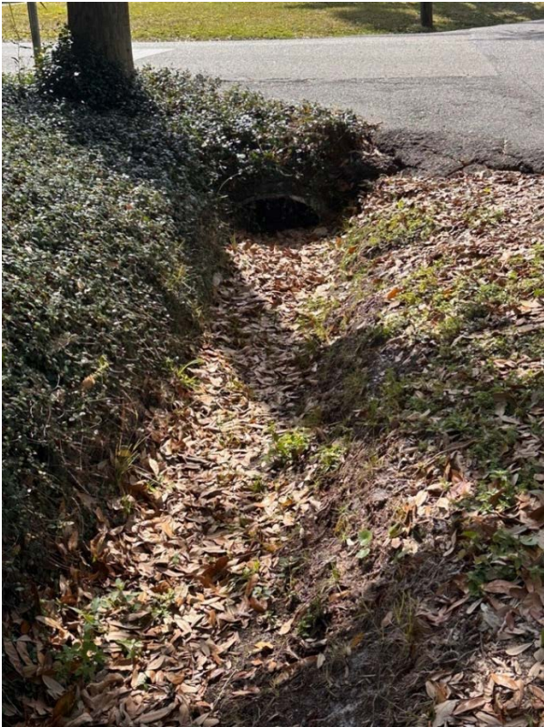
Photo 3-2. Poorly Maintained Drainage Ditch in South of Gandy Source: Jacobs 2024
